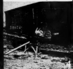
4.—A Barber-Greene "N" Conveyor handling cement from box car to storage. Shown on page 7 of "Contracting with Barber-Greenes."
